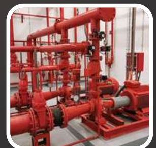
Fire Fighting System
